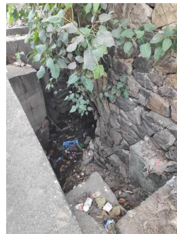
Figure 9:7 Clogged Drains, Vettuthodu
