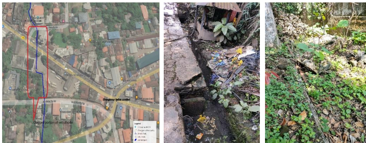
Figure 23:5: Clogged portion of Vettuthodu through KSRTC bus stand & nearby property in Sy no 131
